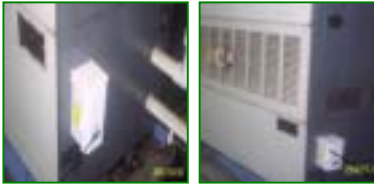
Installed intelligent controllers for air con packaged units
