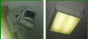
Implemented motion sensors for common staircases, walkways and reception lobby
